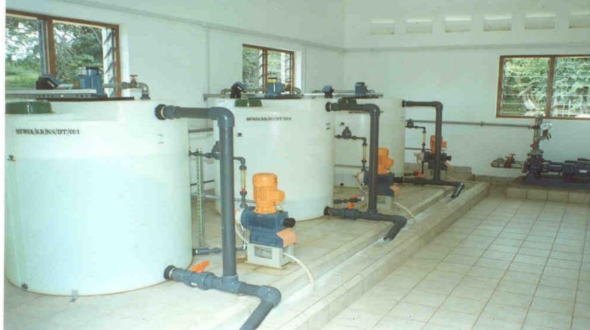
Figure 3: Disinfection facilities at Spring Sources and Reservoirs
